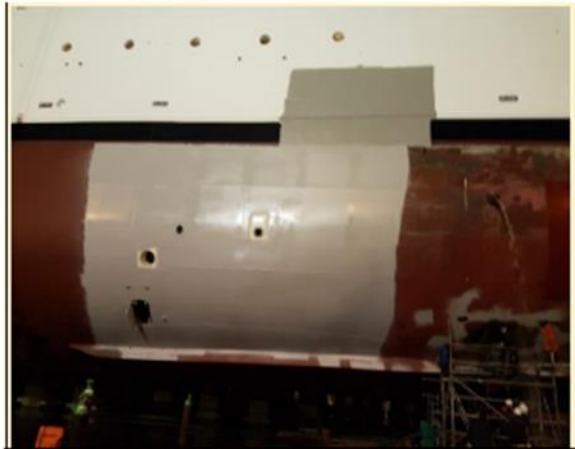
Portside aft view, after full coat application on Vertical Sides (Area Scrubber Scuppers Tank), with INterline 955 white, and with Intergard 7600 grey on Boottop and Topside.
